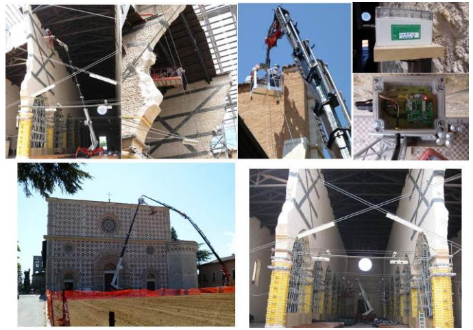
Figure 2. Installation phases of the monitoring system: a) b) sensor positioning on the central walls of the nave, c) sensor positioning beyond the facade, d) f) sensor views, g) on-site testing, h) sensor positioning at the end of the nave walls.
